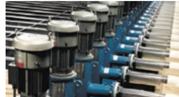
Vertical Pump in Operation
